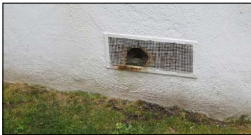
Holes in vent screens are common access points for rodents in buildings.
