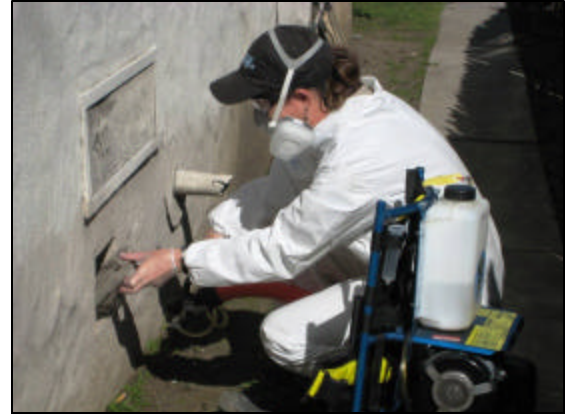
Mosquito Control Technician Kim Keyser removes a vent cover in preparation of a crawl-space mosquito treatment.
