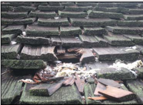
Roof damage caused by a raccoon trying to gain access to the attic
